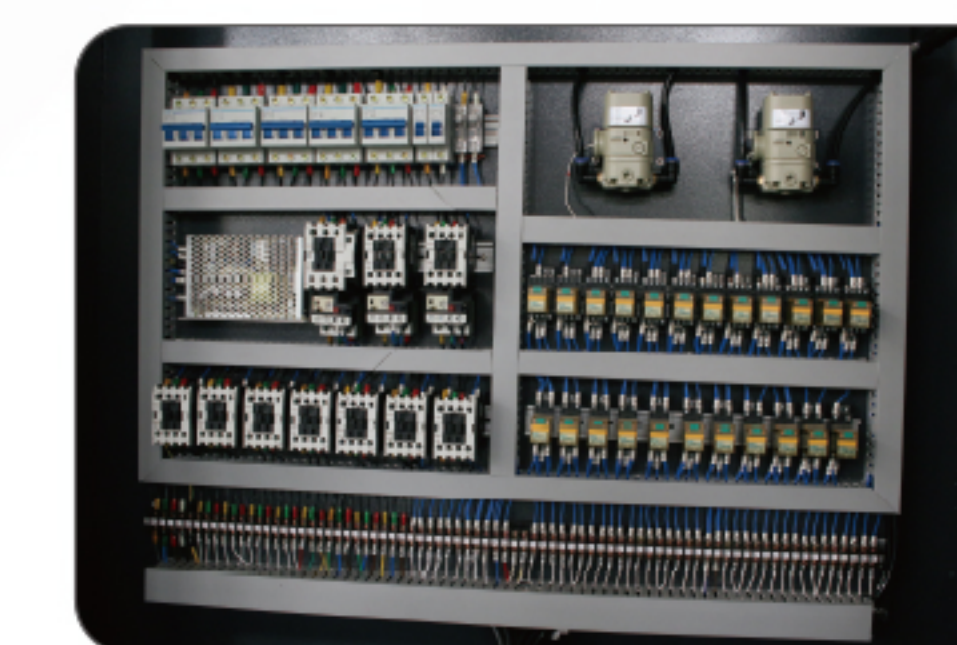
电器设备 Electrical equipment
