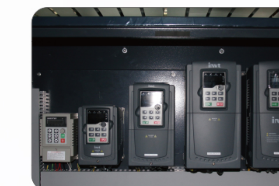
电器操控系统 Electric control system
